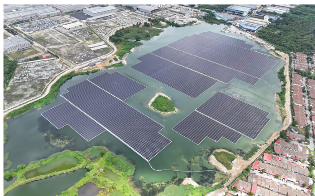
Solar power generation at the Tan Chong Motor
